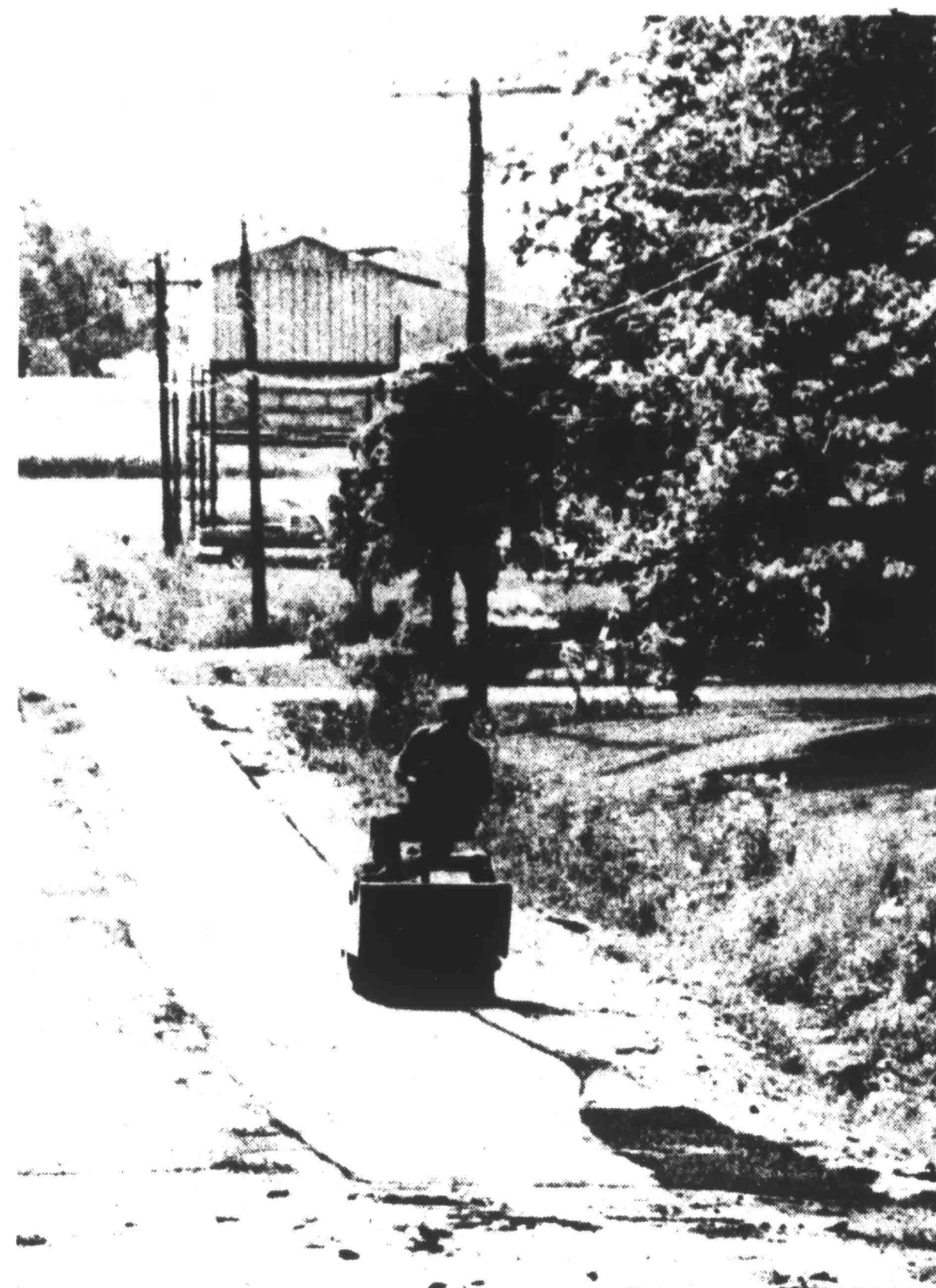
RESIDENTS WERE HAPPY last week as work began on Gates streets to repair damage done while sewers were being installed last year. Mayor John Crutchfield says work should be completed this week.
